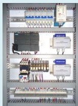
Control cabinet internal view
